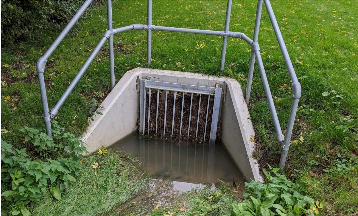
Figure 16 - Culvert screen with internal blockage.
