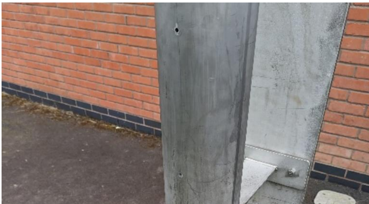
Figure 19 - Small orifices in rainwater pipe.
