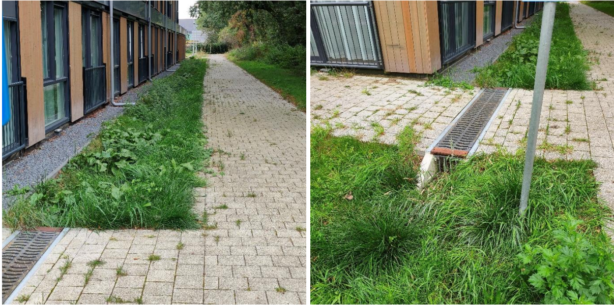
Figure 11 - Rainwater pipes into small-scale swale/filter drain and connection (WCC 2026)
