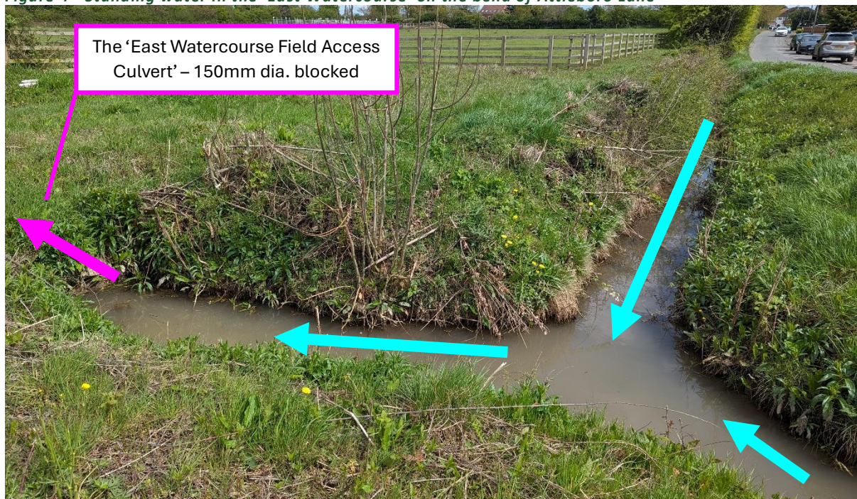
Figure 4 - Standing water in the 'East Watercourse' on the bend of Attleboro Lane
