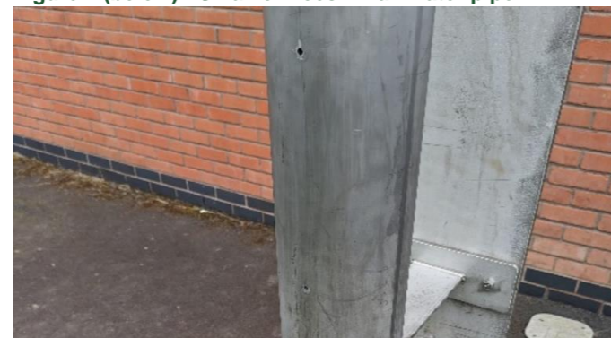
Figure 4 (below) - Small orifices in rainwater pipe
