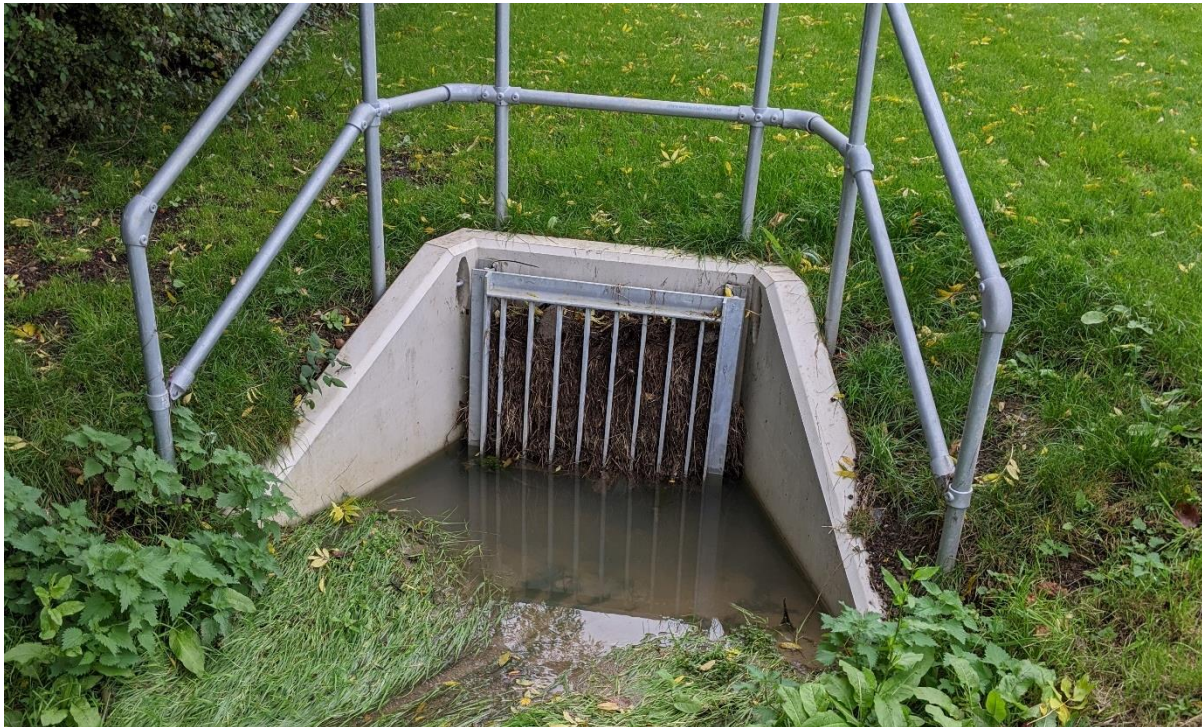
Figure 17 - Culvert screen with internal blockage
