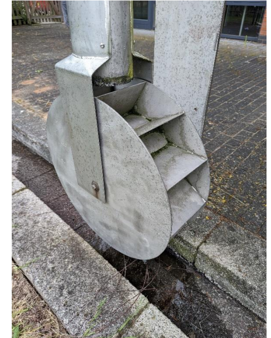
Figure 6 - Water-wheel rainwater pipe outfall
