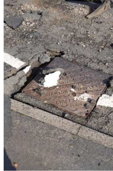
Figure 6 – Damage to surface water sewer manhole cover.
