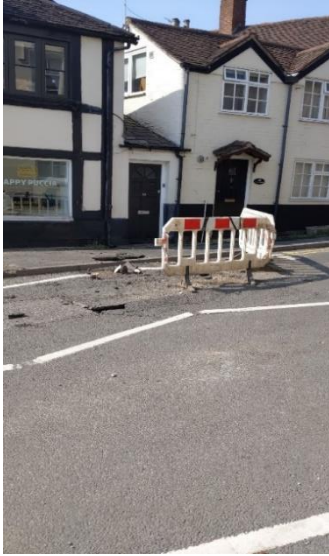
Figure 5 – Damage to highway and manhole cover sectioned off on site visit on 13 th August.
