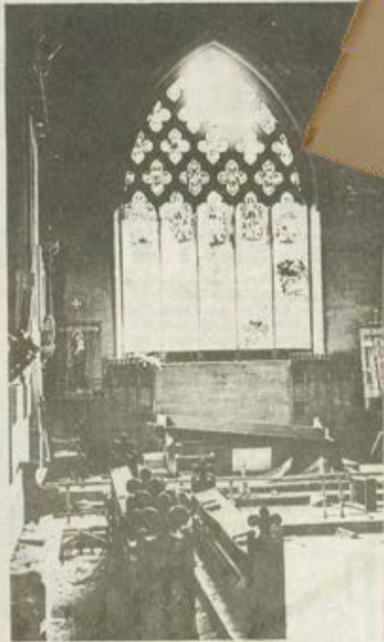
Damage in St Nicolas Parish Church.
