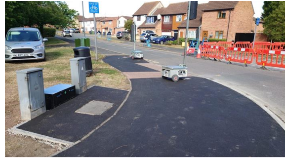
Works completed at Josephs Way, temporary lights in place until installation of the new traffic signal takes place.
