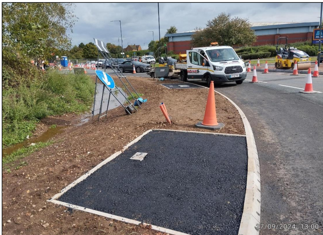
Figure 1 Queensway Roundabout - Traffic Signal Equipment Base Pads
