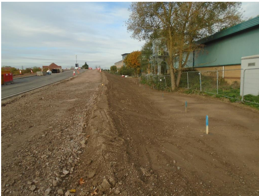
A View of the north-eastern embankment works on the Bermuda Bridge Eastern Approach
