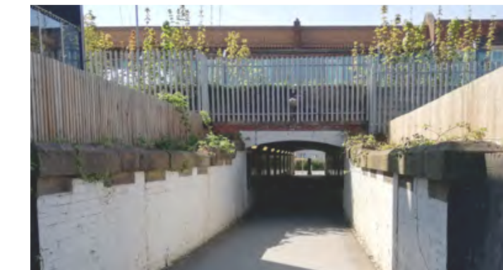
7. Poor quality underpass.
