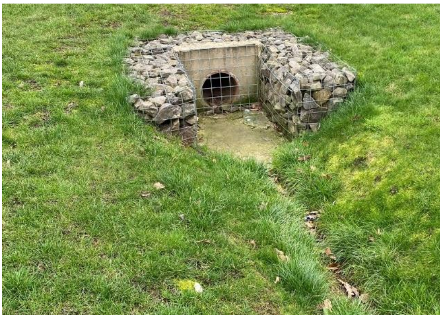
Swale with Gabion headwall at a development in Nuneaton
