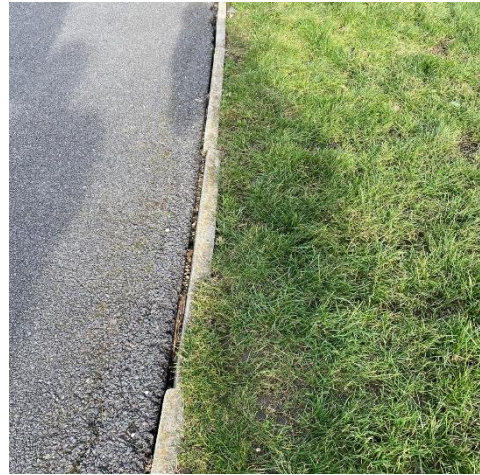
Lack of backing on edging
