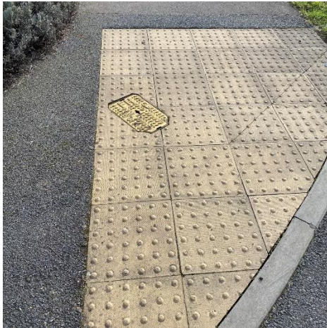
Utility covers should not be placed within the tactiles
