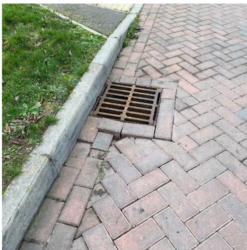
Poor workmanship around gully
