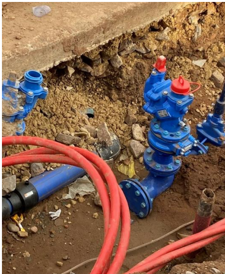
Misplacement of utilities caused undermining of the footway
