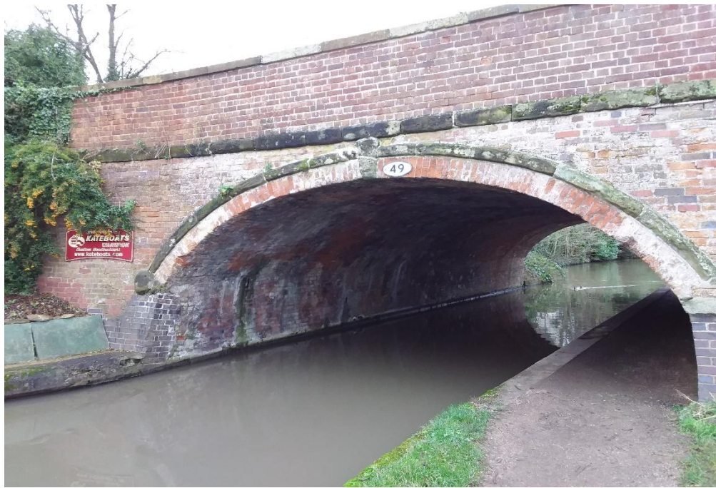
Structure B – A429 road bridge crossing the Grand Union Canal, as seen from the east
